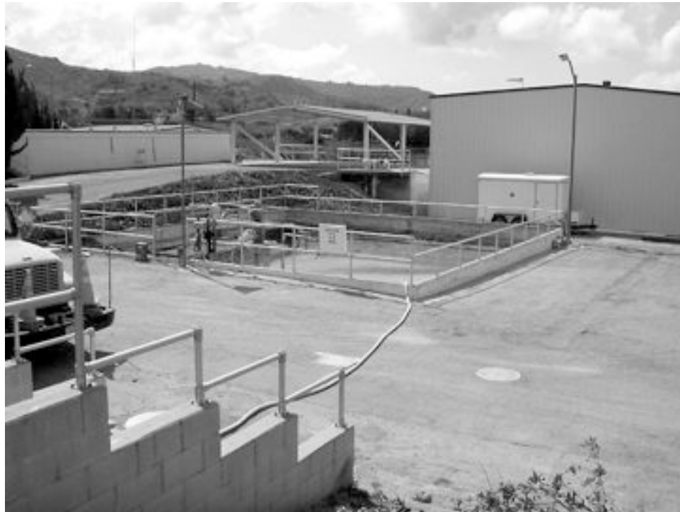
PHOTO 12. Wash Water Basin No. 1, Shops and Storage Building, Sludge Dewatering Unit at rear, facing south (30 April 2002).
