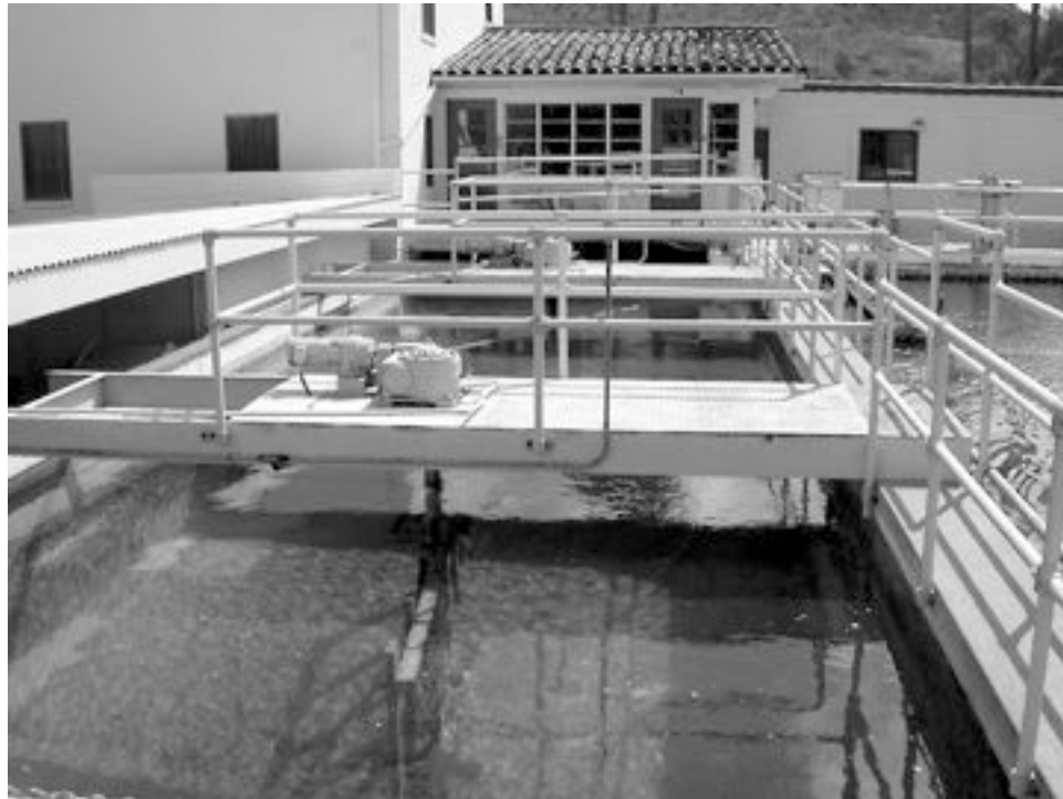
PHOTO 6. Secondary/West Flocculator, facing east (30 April 2002).
