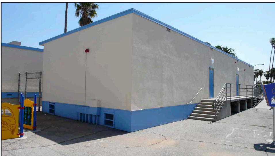
Description of Photo: (View, date, accession #) Photo 260-21. Classroom Building, southern and western elevations. (7 May 2007)
