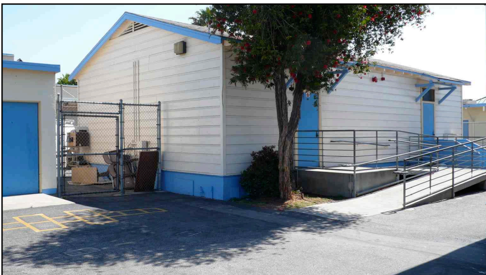
Description of Photo: (View, date, accession #) Photo 290-12. Classroom Building, western and southern elevations. (7 May 2007)
